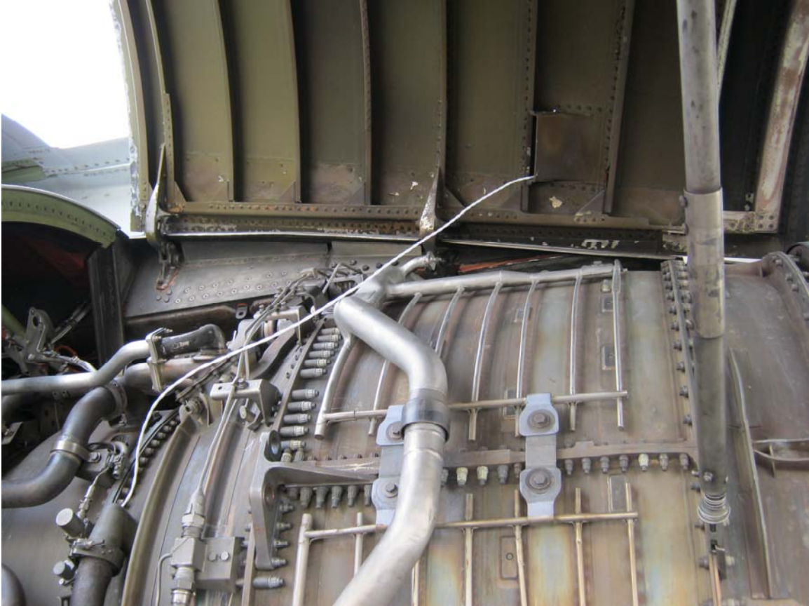
Figure 4. High Temp cable routed from the sensor (lower left in the photo), up and out the vent near the pylon.
